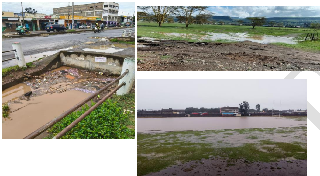
plate 12 - Storm water drainage conditions in Municipality of Gilgil (Kikopey, CBD Drainage, Site, Gilgil Stadium & Ngomongo Estate)
